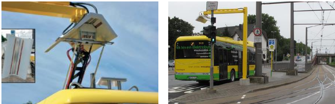
Figure 7 - Pantograph on top of the SOLARIS Bus Roof and Charging Infrastructure at the Station Neumarkt (source: STOAG)
