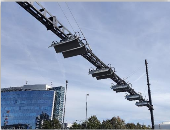
Airport terminus – static charging
